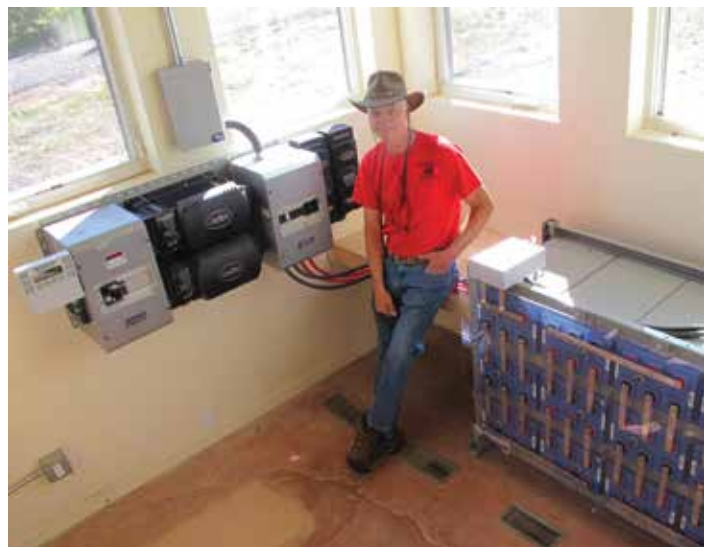
General contractor Kent Marshall takes a break next to the large-capacity energy storage system inside the structure.
